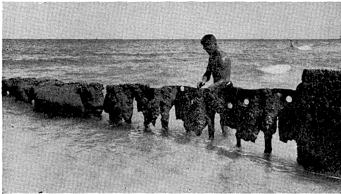
Figure 1—Serious structural deterioration of a groin at Palm Beach, Fla., after 12 years' exposure. The marine life, sabellaria, may be noted.
